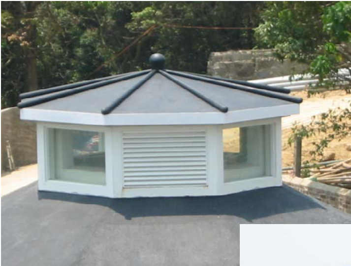
Fiberglass Architectural Roof Cover at Student Hostel of Academy of Performing Arts
